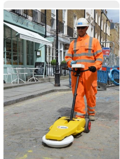
Non-intrusive GPR undertaken on Mottcombe Street without the need for complex road closures on congested routes
