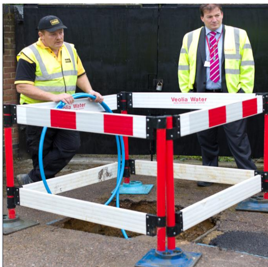
Matthew Rowlatt, Veolia Water Central Director of Community Operations (right), views the demonstration of the Kobus Pipe Puller at Veolia’s permanent Pipe Pulling Test Site in Luton.
